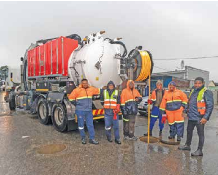
Pricey and preventable: The City's teams have their hands full keeping the sewer system in Dunoon clear of objects that do not belong there. Abuse of the sewer system is consuming far too much of the City's time and taxpayers' money.
